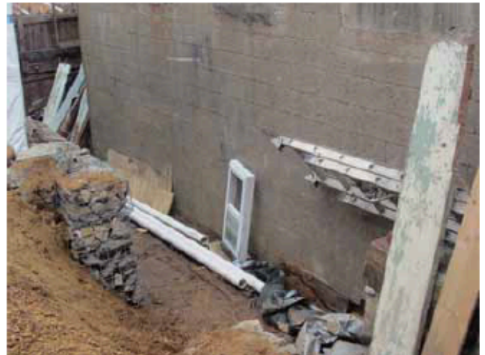
BELOW: Construction of a new fire escape behind Artisan Tattoo begins; a recent building inspection requires compliance with all ADA standards in order for the business to keep its doors open. Photo by Andrew McKeon.
